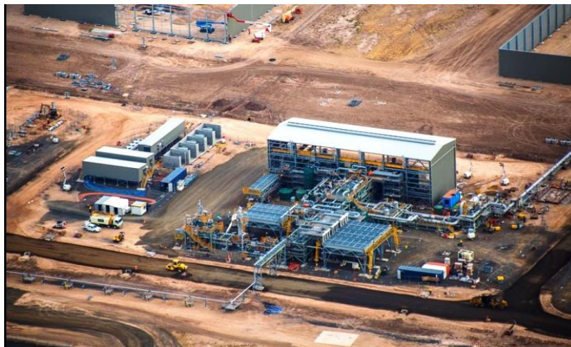
Figure 2 APLNG Gas Processing Facility, Reedy Creek
